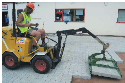
A hydraulically operated clamping system is used to lift a 'cluster' of blocks already in the required laying pattern.
