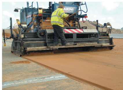
The laying course can also be placed particularly efficiently with a paver machine. A sonic sensor (on the left of the photo) controls the screed box to ensure a constant thickness.
