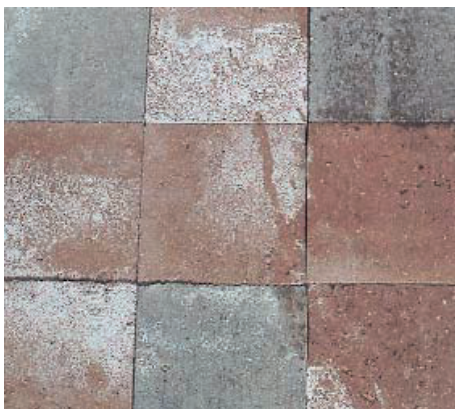
Block paving showing efflorescence
